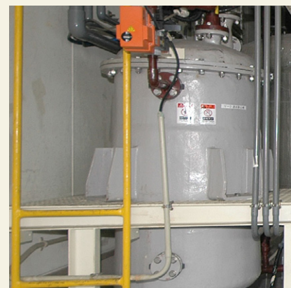
過水除去槽 Reactor for hydrogen removal
