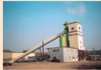
for aggregate (ready-mixed concrete plant)
